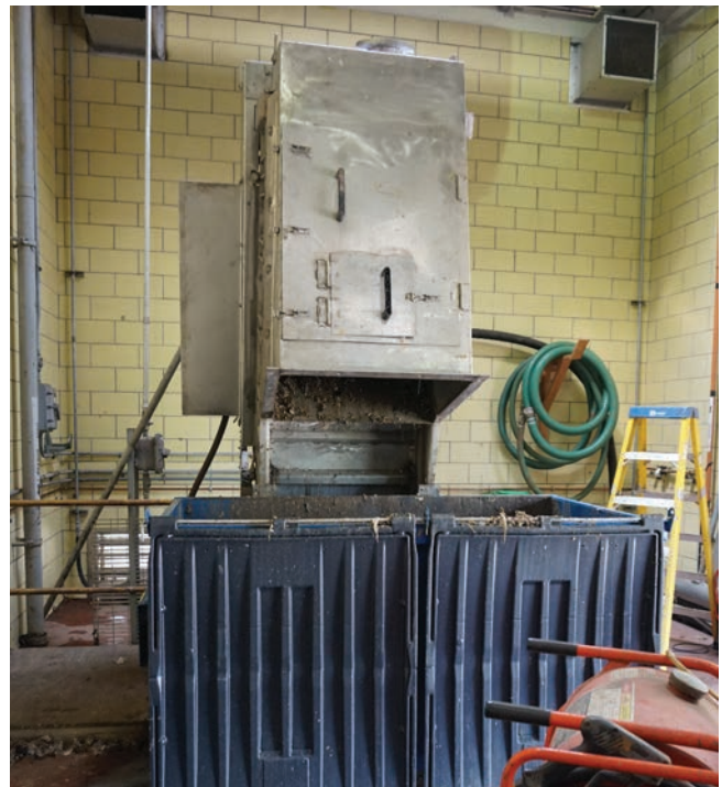
Thanks to the Lock Link screen, a 3 cubic yard dumpster replaced the bucket.
